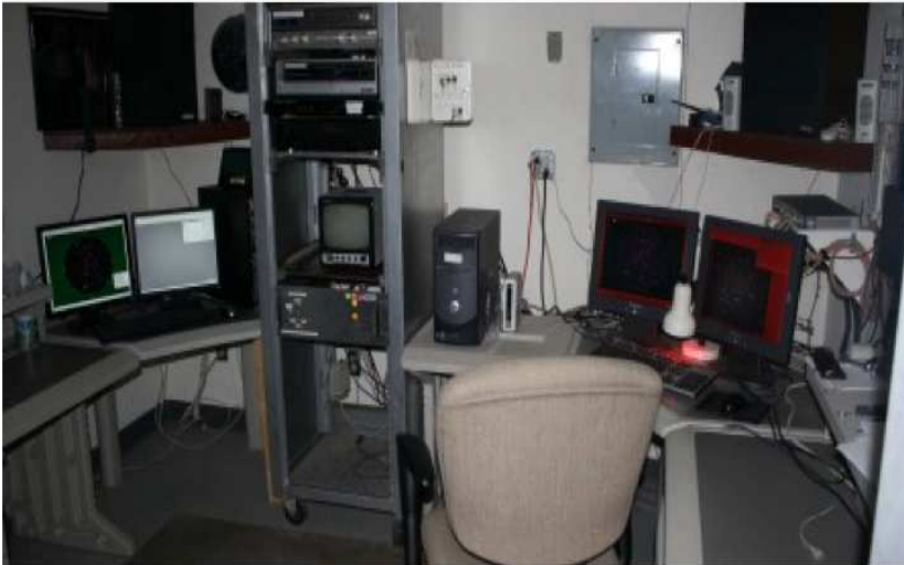
Roll-Off Control Room
